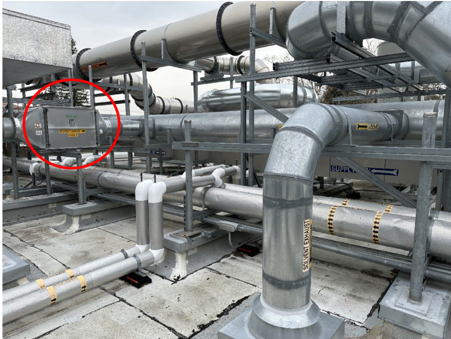
Photograph 11b (IMG_5589.JPG - 01/16/24): A photo of Apple's solvent exhaust system on the right (B(4)) emerging from the ceiling in the B(4) Area and connecting to the larger exhaust system piping on the roof. The "Activated Carbon" box for B(4) is located on the left side of the photo, which is used to vent VOCs.
