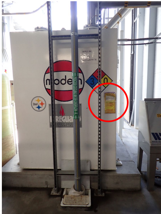
Photograph 6a (P8170051.JPG - 08/17/23): A photo of Apple’s 1,700-gallon stainless-steel hazardous waste tank. The tank was marked with the words, “Hazardous Waste” and used for the accumulation of spent solvent waste. At the time of the inspection, the solvents were being managed as California Only Waste.
