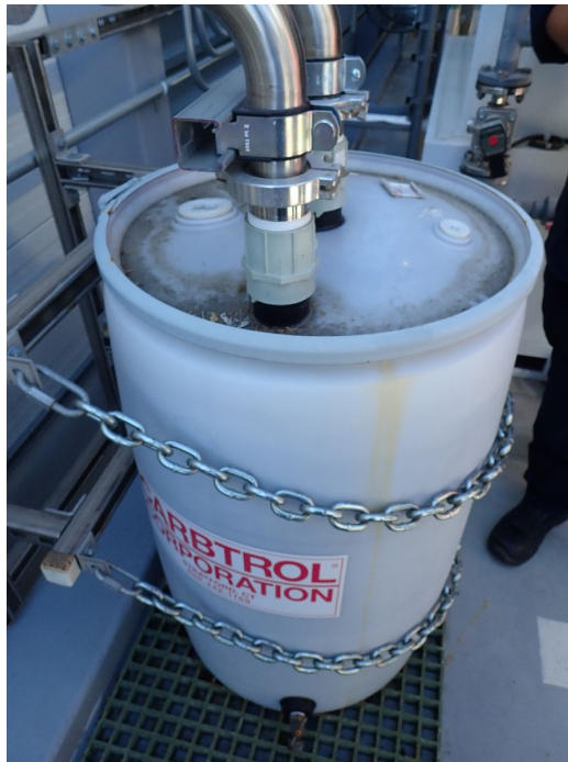
Photograph 7a (P8170062.JPG - 08/17/23): A photo of a 55-gallon container filled with “Activated Carbon” and located on the roof of Building 1. This drum is used to capture the VOC emissions from Apple’s 1,700-gallon spent solvent waste tank. The container was not labeled or identified in Apple’s air permit or their RCRA tank assessment.
