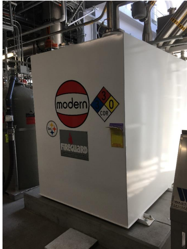
Solvent Waste Tank (SW-TNK-2) (2018 Photo)
