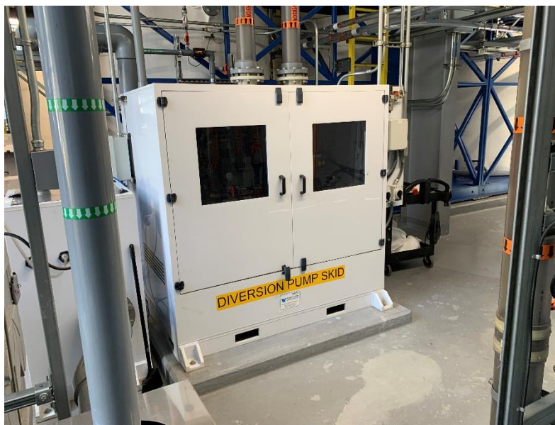
Diversion Pump Skid and Ancillary Piping
