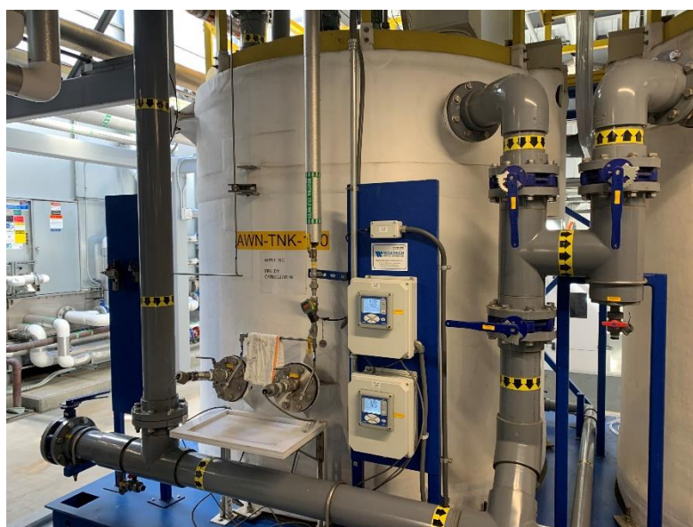
Reaction Tank (AWN-TNK-100) and Ancillary Piping
