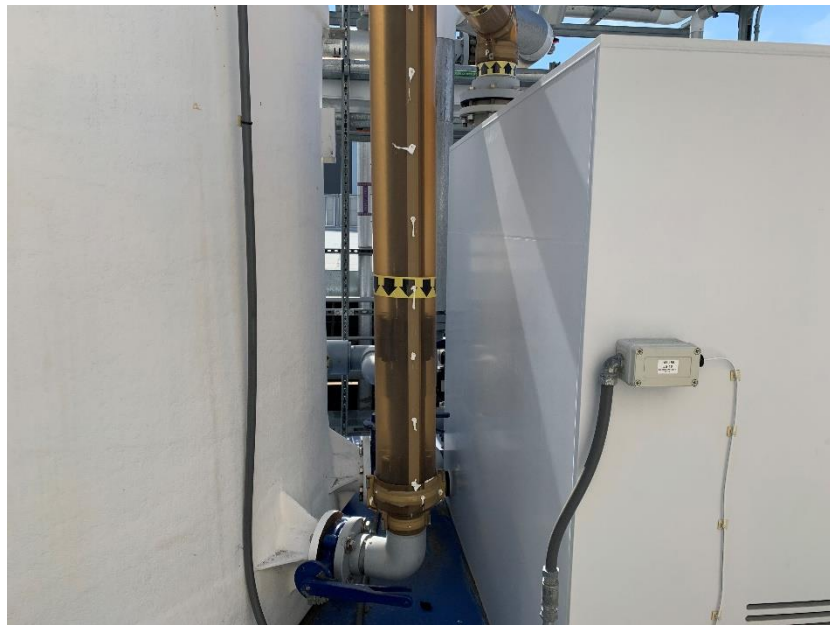
Ancillary Piping to Equalization Tank
