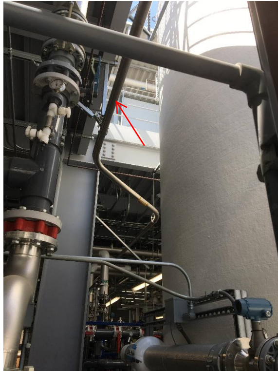
Ancillary Piping (2018 Photo)
