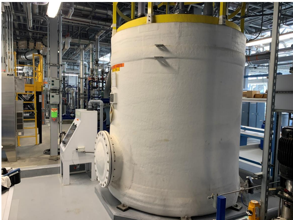
HMC-TNK-2 and piping to Heavy Metal Concentrate Pull Station (HMC-TFS-1)
