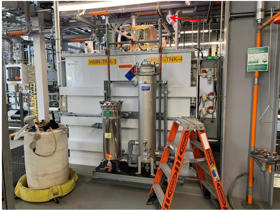
HMR-TNK-3&4 and piping to Vacuum Distillation Evaporator (VDE-1)
