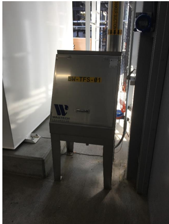
Solvent Waste Tank Pumpout Cabinet (2018 Photo)
