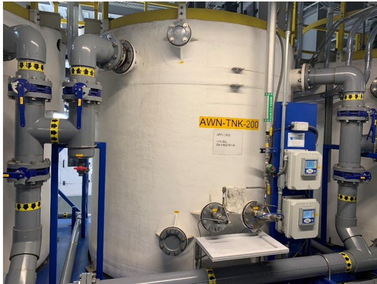
Reaction Tank (AWN-TNK-200) and Ancillary Piping
