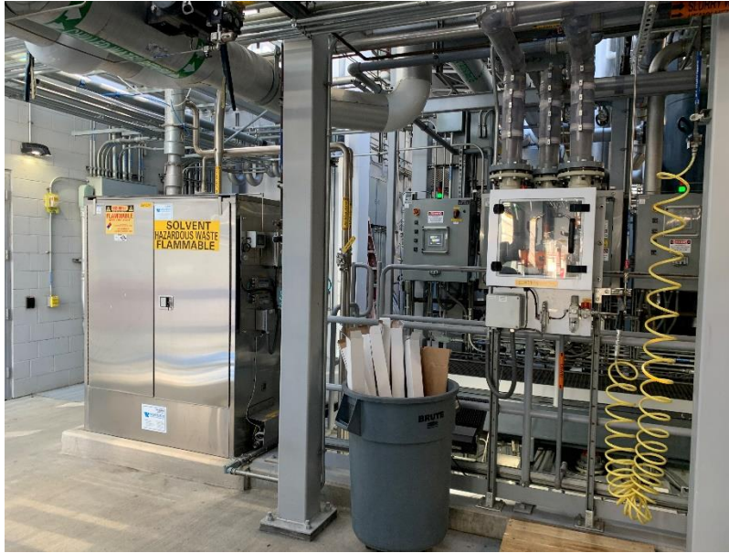
Solvent Waste Collection Cabinet (SW-CC) and Ancillary Piping
