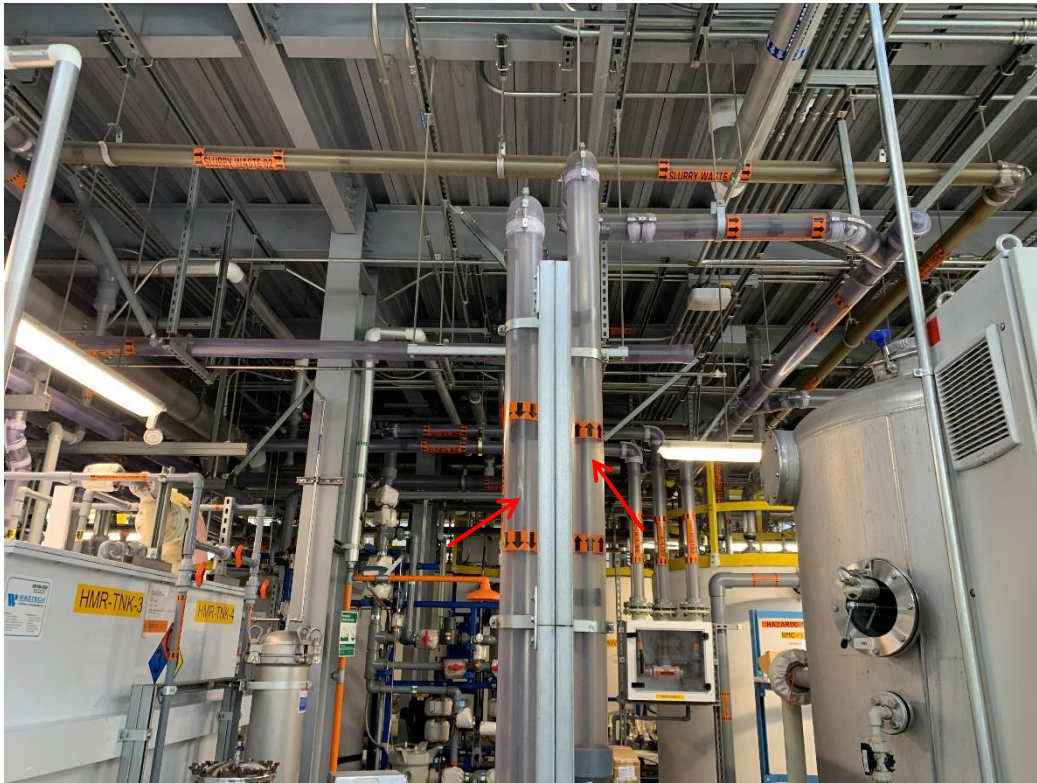
Piping to VDE-1 (left) and piping to HMC-TNK-2 (right)
