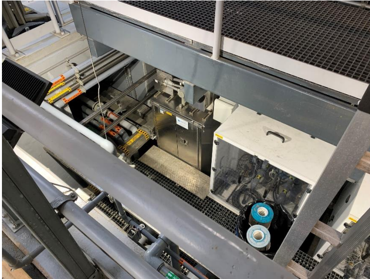
Solvent Waste Lift Station (SW-LS) and Ancillary Piping
