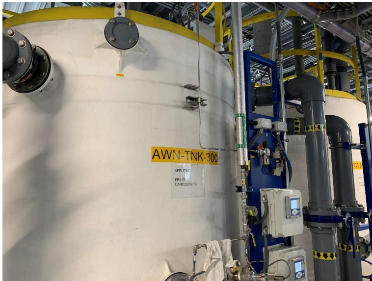
Reaction Tank (AWN-TNK-300) and Ancillary Piping
