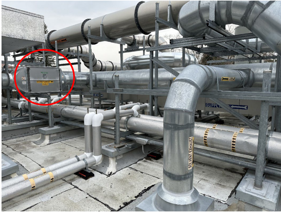
Photograph 11b (IMG_5589.JPG - 01/16/24): A photo of Apple's solvent exhaust system on the right ( B(4) ) emerging from the ceiling in the B(4) Area and connecting to the larger exhaust system piping on the roof. The "Activated Carbon" box for B(4) is located on the left side of the photo, which is used to vent VOCs.
