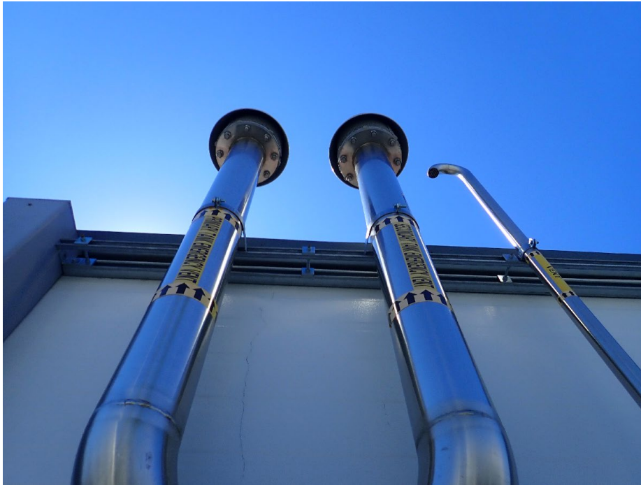
Photograph 7b (P8170061.JPG - 08/17/23): A photo of three vents connected to Apple’s 55-gallon container filled with “Activated Carbon”. The two vents on the left are emergency vents for the double-walled tank. The vent on the right is the main vent.
