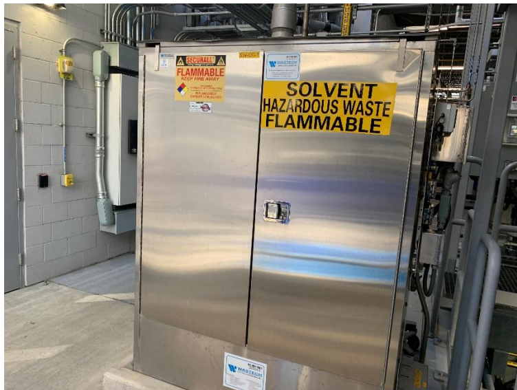
Solvent Waste Collection Cabinet (SW-CC)
