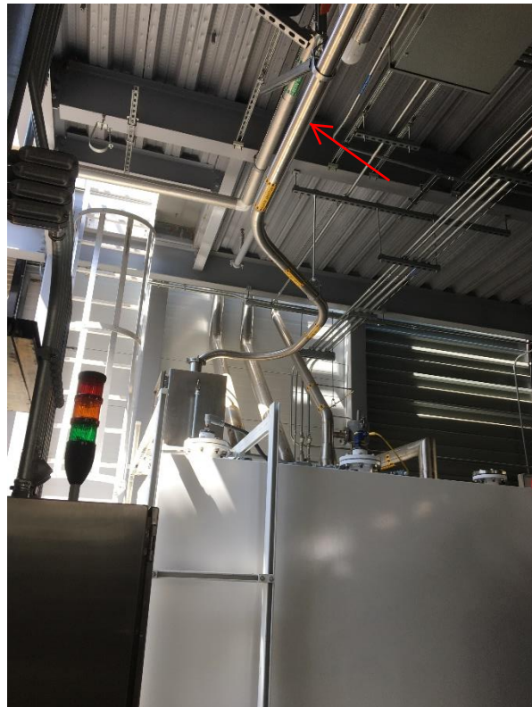
Ancillary Piping (2018 Photo)
