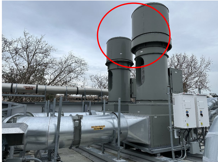
Photograph 11c (IMG_5591.JPG - 01/16/24): A photo of Apple's solvent exhaust piping connecting to one of the main general exhaust systems on the roof of Building 1. The general exhaust system vents the air directly to the atmosphere.
