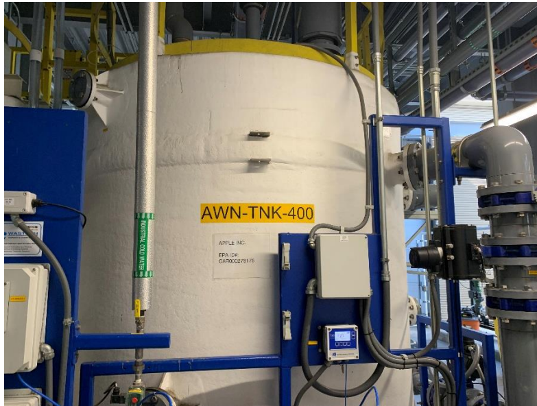
Diversion Tank (AWN-TNK-400) and Ancillary Piping
