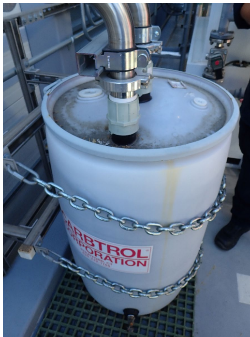
Photograph 7a (P8170062.JPG - 08/17/23): A photo of a 55-gallon container filled with “Activated Carbon” and located on the roof of Building 1. This drum is used to capture the VOC emissions from Apple’s 1,700-gallon spent solvent waste tank. The container was not labeled or identified in Apple’s air permit or their RCRA tank assessment.
