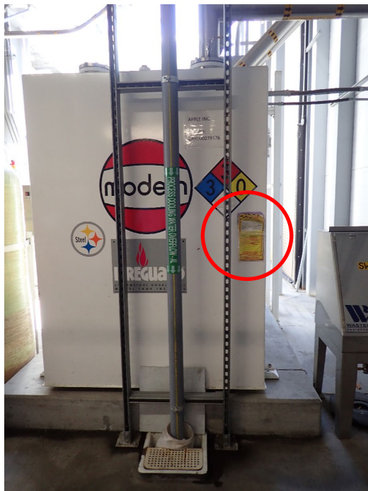
Photograph 6a (P8170051.JPG - 08/17/23): A photo of Apple’s 1,700-gallon stainless-steel hazardous waste tank. The tank was marked with the words, “Hazardous Waste” and used for the accumulation of spent solvent waste. At the time of the inspection, the solvents were being managed as California Only Waste.
